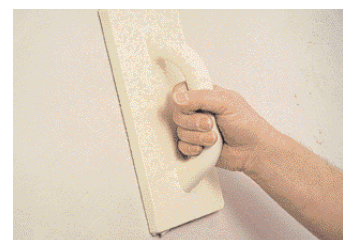
... and – once it has just started to set – leveled with a trowel
